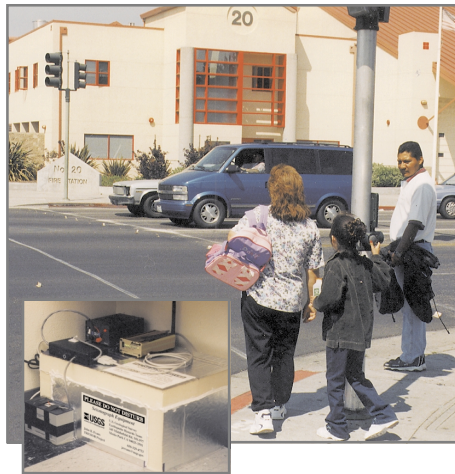
The U.S. Geological Survey, as part of a public-private partnership, operates a network of seismic instruments at many sites in Oakland, California. The instruments, such as this one (see inset) in Fire Station 20, measure and report levels of ground shaking. This network will help guide emergency response to areas most in need in future quakes.
